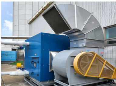
Hotel – Free Cooling System
